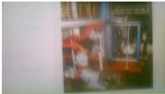
Circulating pump and heat exchanger
