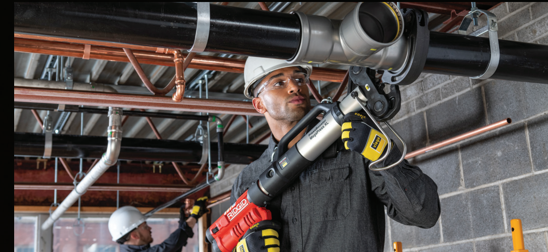
Secure, flameless connections on gas lines
