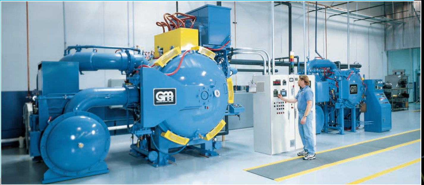
MODERN VACUUM HEAT TREATING FACILITY
