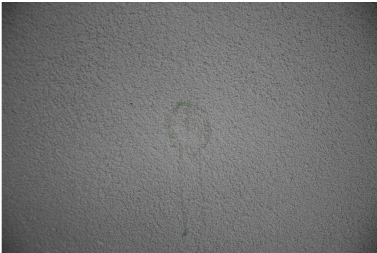
Picture 7: Inspection of the damage caused by the impact - only a slight depression is visible on the surface of the ETICS, without any cracks
