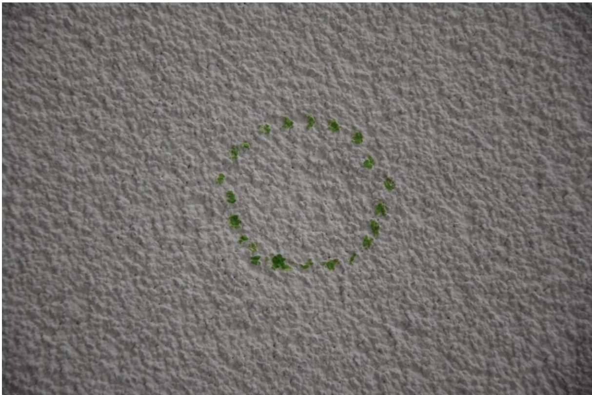
Picture 10: Inspection of the damage after the impact - almost no visible damage on the surface of the ETICS
