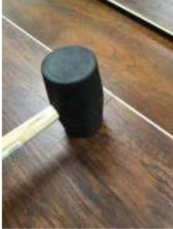
Incorrect (on the seam)
