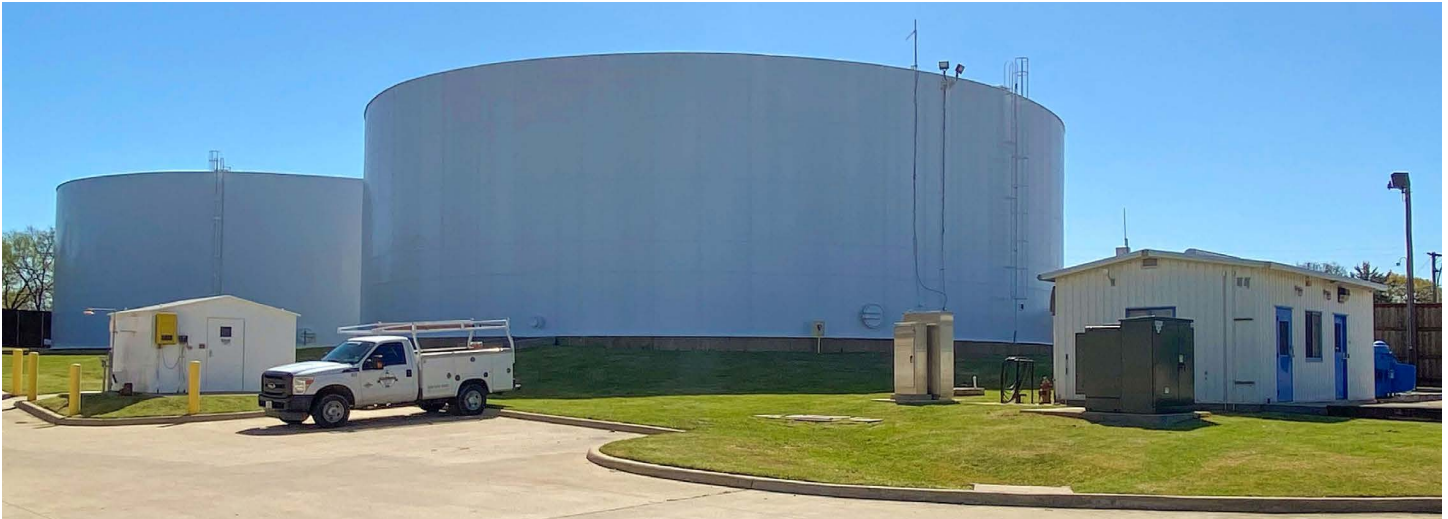
ONE WAY THE DISTRICT SUPPLEMENTS WATER DELIVERY IS WITH TWO 3 MILLION GALLON GROUNDWATER STORAGE TANKS.
