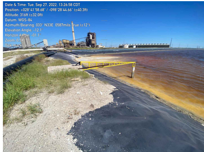
7323 - Facing North. South Equalization Basin Water Level Gauge.
