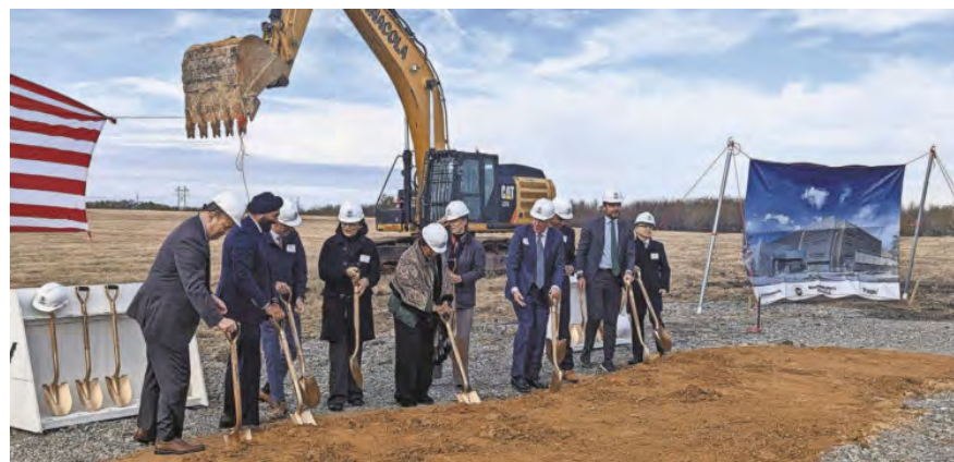
Officials ceremoniously toss dirt during the groundbreaking ceremony for the new $5 billion GlobalWafers site Thursday. Michael Hutchins
