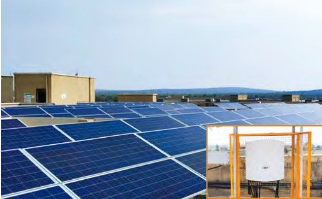
Police Training Project, India 450kW
