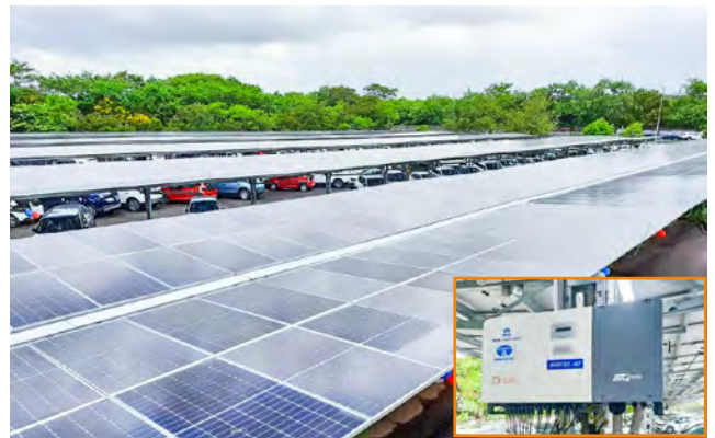
Carport project, India 6.2MW
