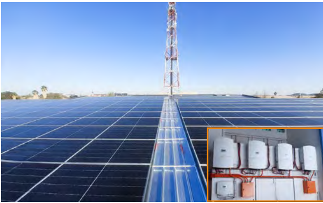
SolWorx Project, Namibia 272kW
