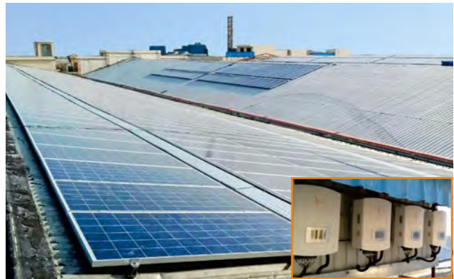
RSWM, India 3.6MW
