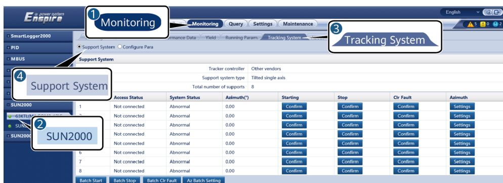
Figure 6-24 Support system (tracking system)
