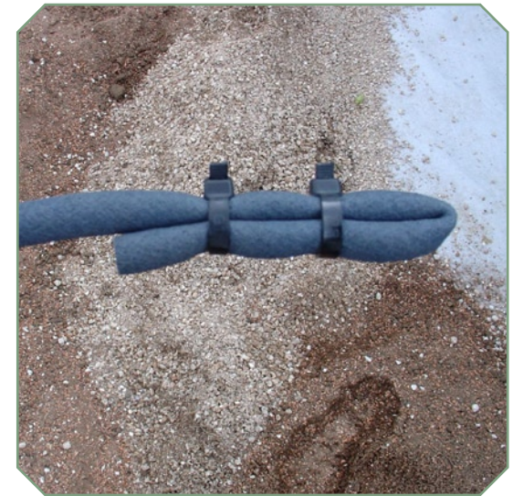
Leaky pipe end showing cable ties
