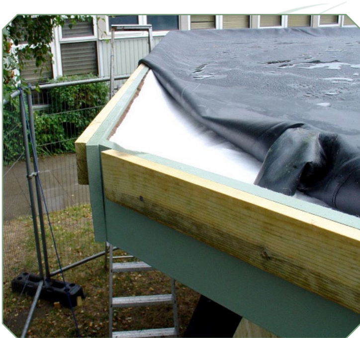
75mm spacer fixed flush with top of fascia and butyl outlet sleeve ready to pull through lower geotextile and roof deck
