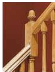
Handrail runs straight into the top block of the newel post at all landings.
