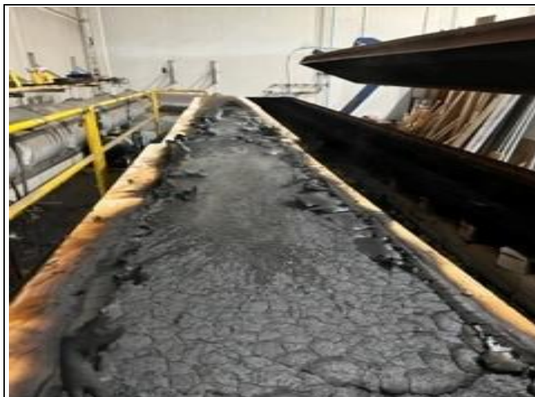
Photo No. 2 Post Test
