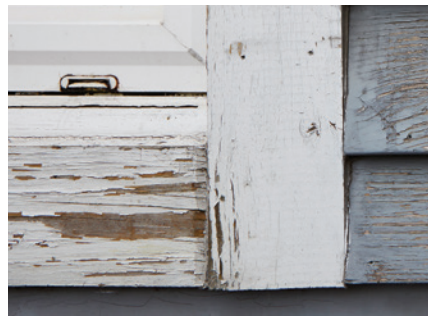
PAINTED WOOD Paint needs constant repainting.
