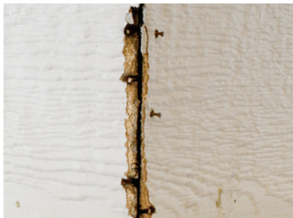
ENGINEERED WOOD Unsealed ends? Rot is coming.
