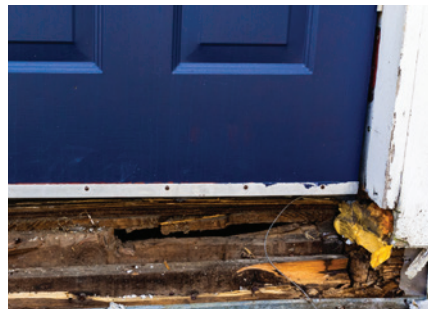
PAINTED WOOD Moisture cycles destroy wood.
