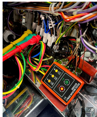
Phase rotation meter connected to supply terminal, accessed through front of unit
