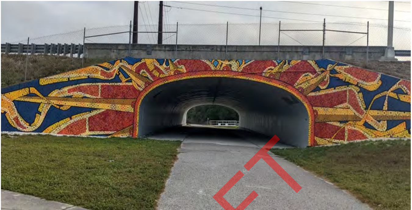
Figure 25. Underpass with public art enhancement and width to enhance natural lighting and safety
