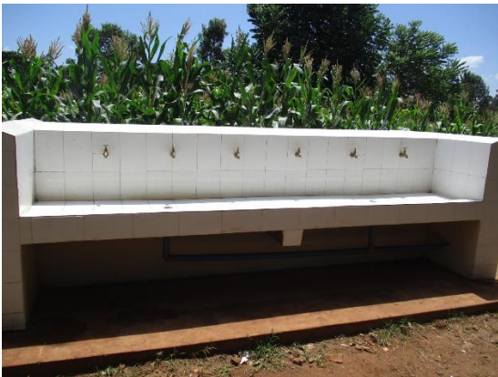
Washing sink at Ayalagaya Secondary School
