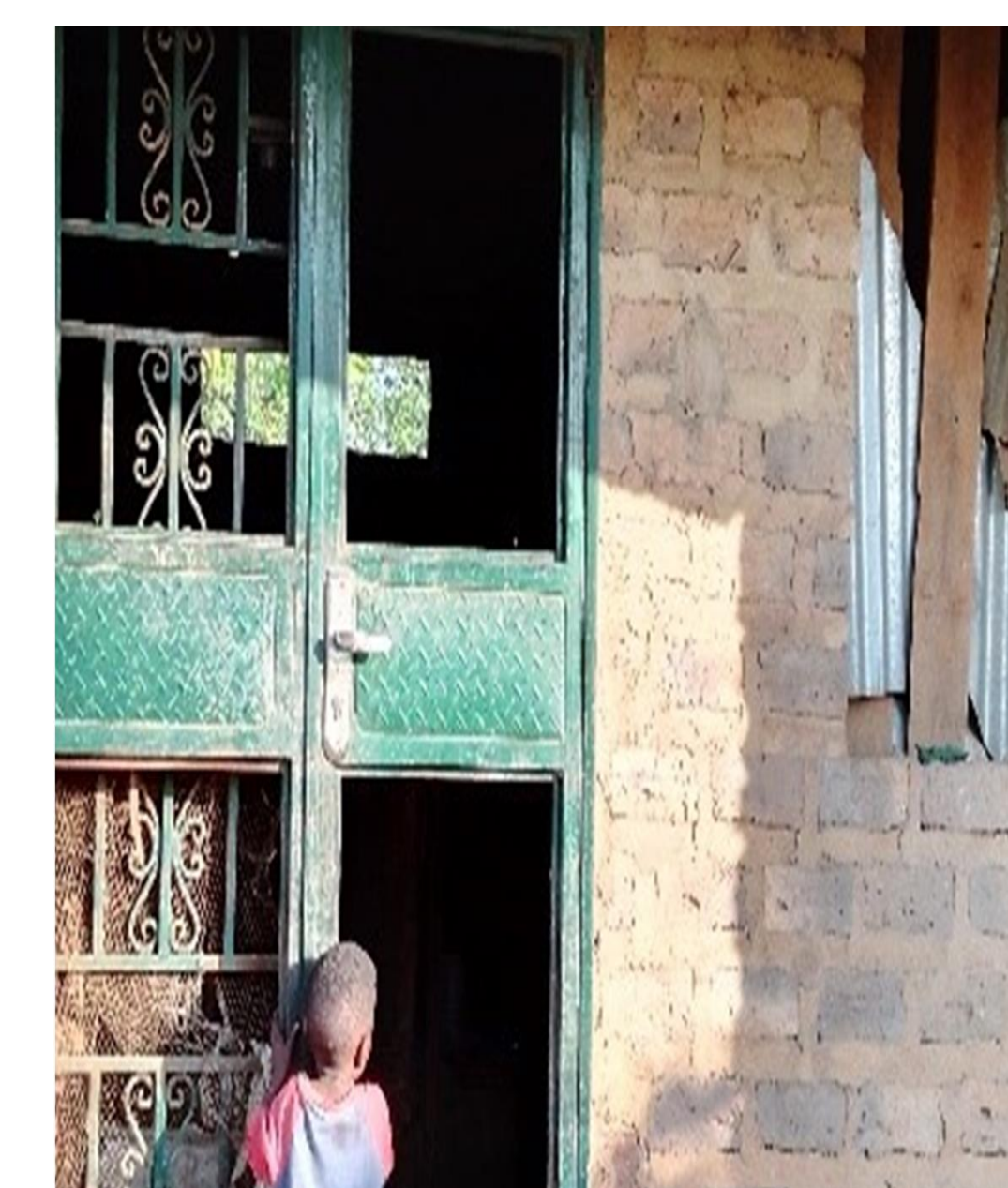
Poor housing with no window and door panes.
