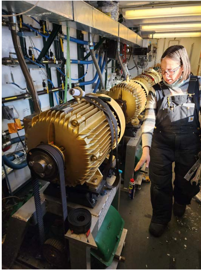
Figure 15: Four Myers pumps (green) and Baldor motors (gold) inside the High Pressure Pump building.
