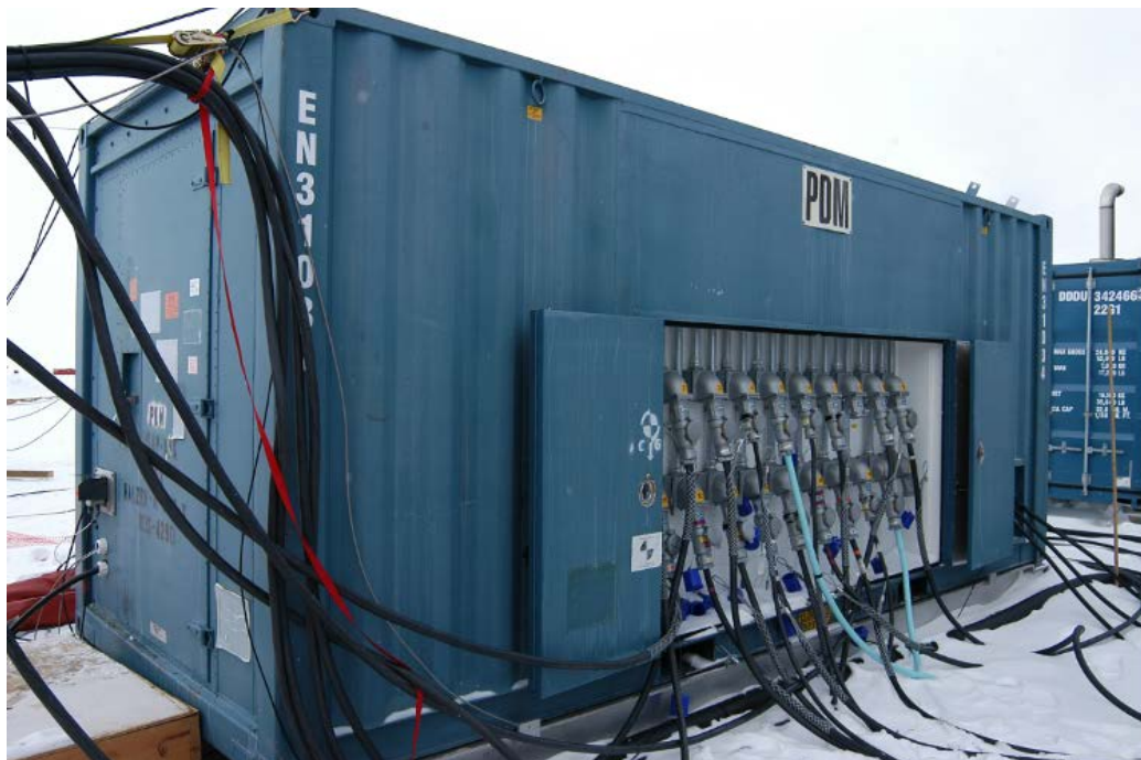
Figure 9: The Power Distribution Module distributes all of the electrical loads to the Seasonal Equipment Site and Tower Operations Site.
