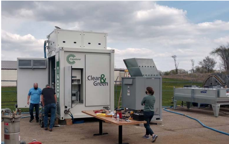
Figure 7: A Capstone CS1000S microturbine has been purchased by PSL and is currently being used for research and development and testing in support of IceCube-Gen2. The microturbine is currently installed in the PSL testbed.
