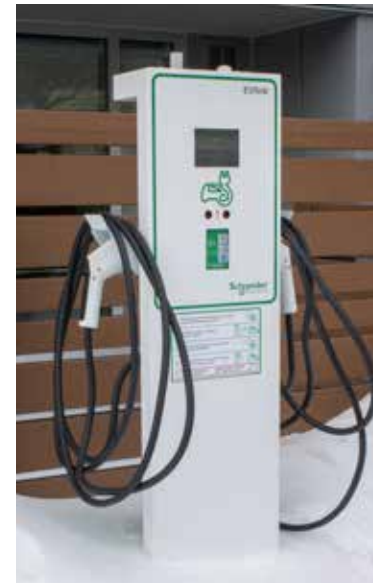
Electric Car Charging Station
