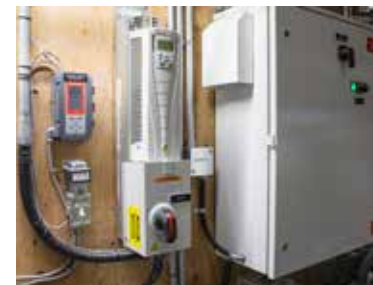
Variable Speed Drive for Make Up Air
