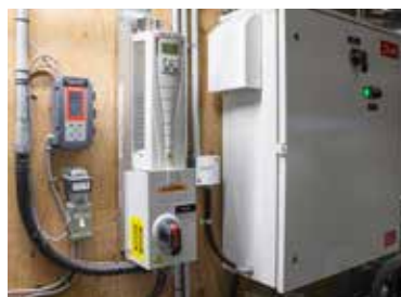
Variable Speed Drive for Make Up Air
