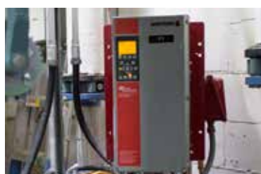
Variable Speed Booster Pump
