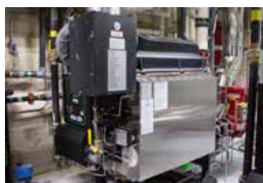
High Efficiency Boiler
