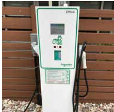
Electric Car Charging Station
