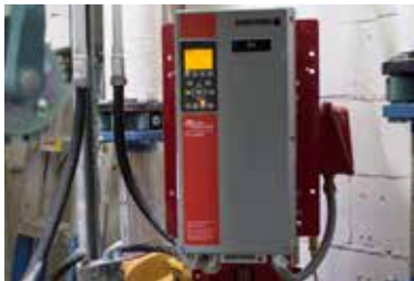
Variable Speed Booster Pump
