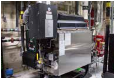
High Efficiency Boiler
