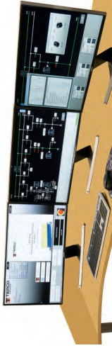
PST2250-15 SCADA System
