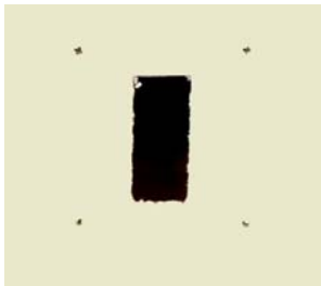
Fig.7: The four (4) outside mounting holes have been marked and the rectangular center opening has been traced and removed from the wall. The four (4) drywall anchors have been inserted into the wall.
