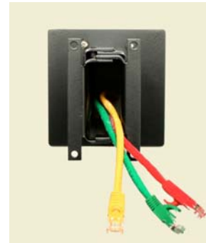
Fig.9: The three Cat-5e cables have been pulled through the Adjustable Extension Mount. The mount has been attached to the wall anchors with four (4) #8 Screws.
