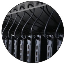
OVERHEAD WIRE MANAGEMENT
