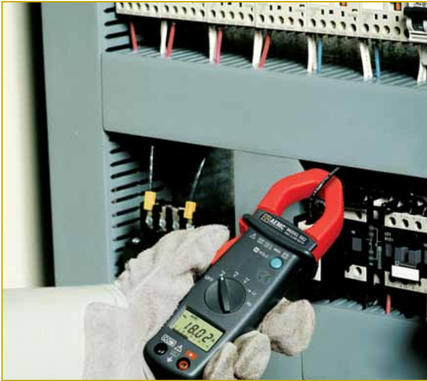
Model 502 monitoring phase current on a power panel.
