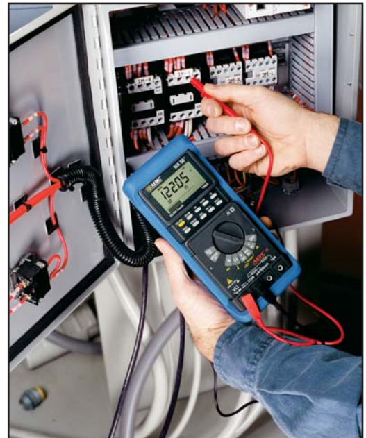
Model MX56 III measuring DC voltages in a signal control panel.
