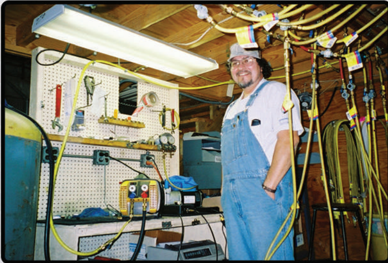
Above: At times running 8-10 hours a day, 5 days a week, the G5Twin has proven to be extremely fast and reliable. Not a problem, thanks to the G5Twin.
