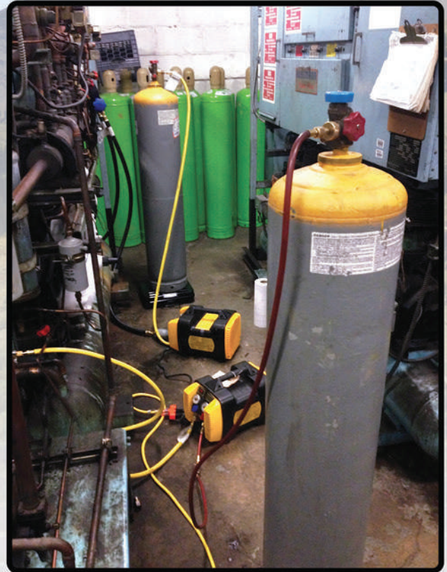
Above: On an R407A system retrofit of a low temperature ice cream case, the G5Twin recovered 600 pounds of R22 in record time, using the push-pull method.
