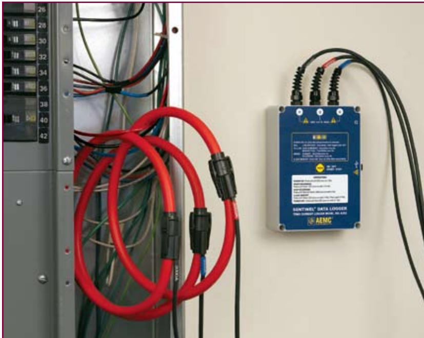
The Model SDL A302 recording AC current on a three-phase power panel.
