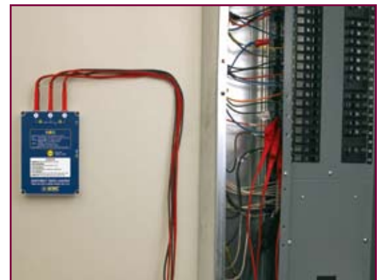
Model SDL V301 recording three-phase voltage on a lighting panel.
