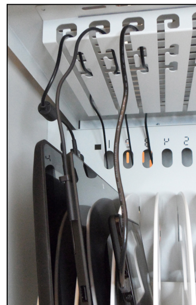
Cable management channel
