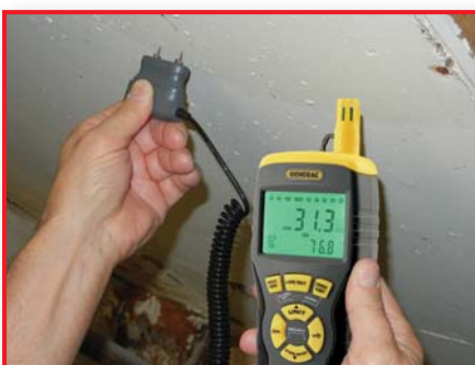
Locate moisture/water damage
