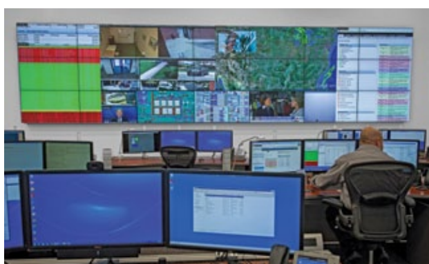
▲ American Water's control room display wall comprises 21 ultra-narrow bezel LCD flat panels from Christie.
