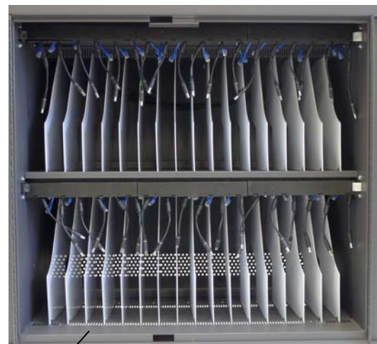
Inside view of notebook compartments with network and power connections
