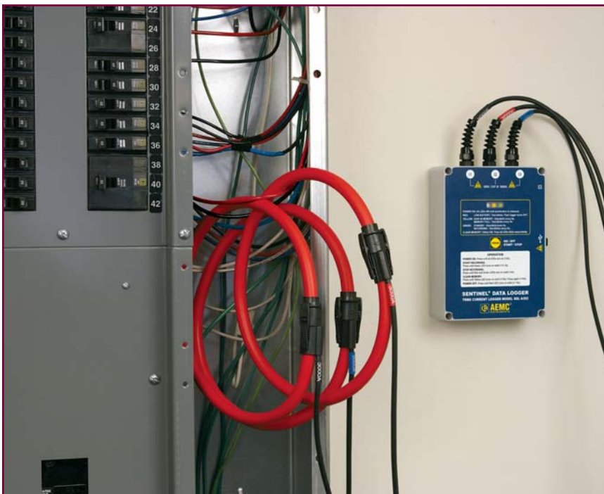
Model SDL A302 three-channel current logger monitoring lighting loads.
