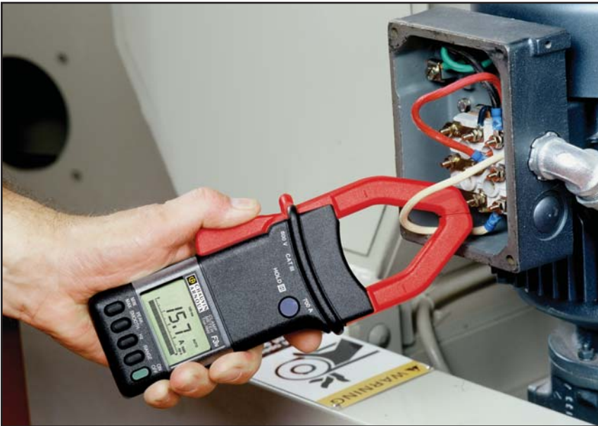
Model F3N measuring phase current on a 3 phase motor.
