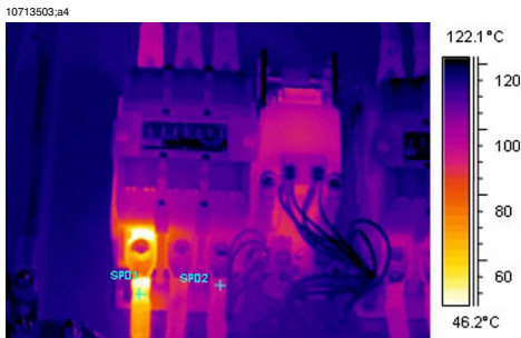
Figure 16.9 An infrared image of indoor electrical equipment (2)
