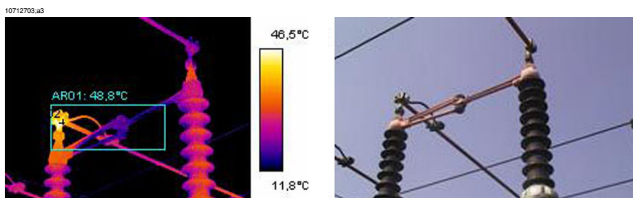
Figure 16.1 An infrared and a visual image of a power line isolator
