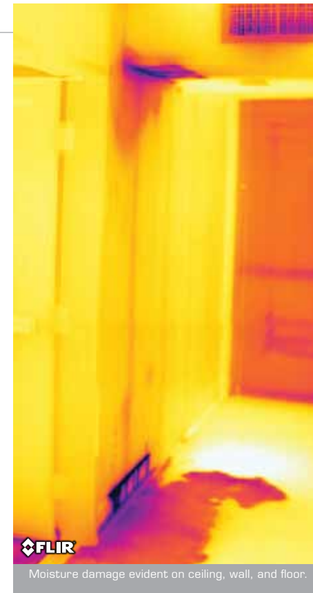
Building Diagnostics Even small areas of moisture intrusion can be easy to spot with an infrared camera. Locate and repair hidden water damage before a trickle turns into a flood.
