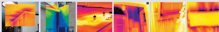
Water Damage — Water leak on ceiling, gutter, and roof top
