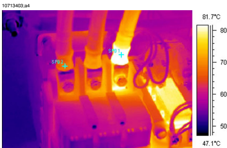
Figure 14.8 An infrared image of indoor electrical equipment (1)
