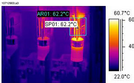
Figure 14.3 An infrared image of a fusebox where the maximum temperature is displayed
