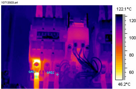
Figure 14.9 An infrared image of indoor electrical equipment (2)
