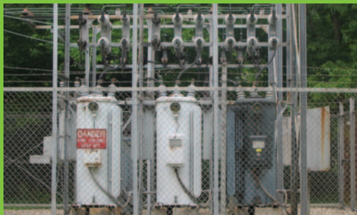
Examine transformers, comparing similar connections under similar loads.
