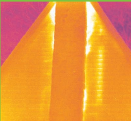
Inspecting to locate air leakage requires a 4°F or higher temperature difference between inside and outside air, in order to get accurate readings. Air leakage can be into the building, as in the cold air shown leaking through the floor, or out of it, as in the warm air leaking out alongside the chimney. Images courtesy of Snell Infrared ©2005
