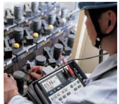
3551 Checking the battery in an Uninterruptible Power Supply (UPS) without shutting down
