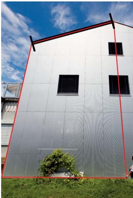
The trapezoid function provides you with a simple way of measuring roof slopes.
