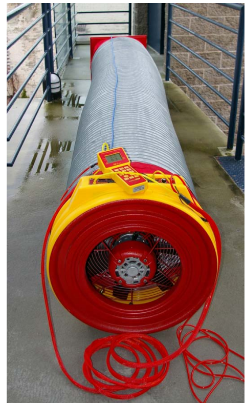
Figure 32. Flex Duct attached for calibration.
