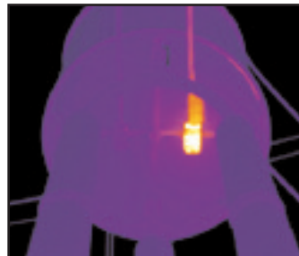
Overheat in power transformer
