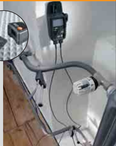
Inspects flow/return temperature
