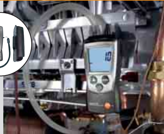
Differential pressure measurement on a gas heater
