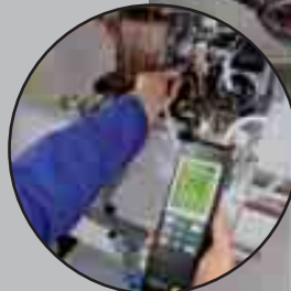
Checking the gas connection pressure and gas flow pressure as well as adjusting the jet pressure.
