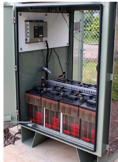
Installation to 48V Switchyard Battery
