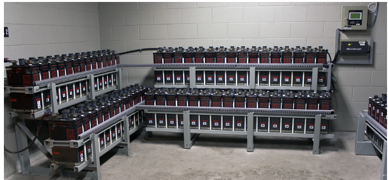
iPQMS Installation on 125VDC Utility Battery System
