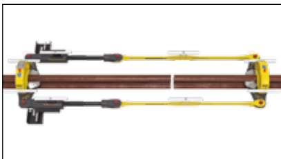
▲ Modular 70 ton stressor and holds the rail in neutral length during the welding process.
