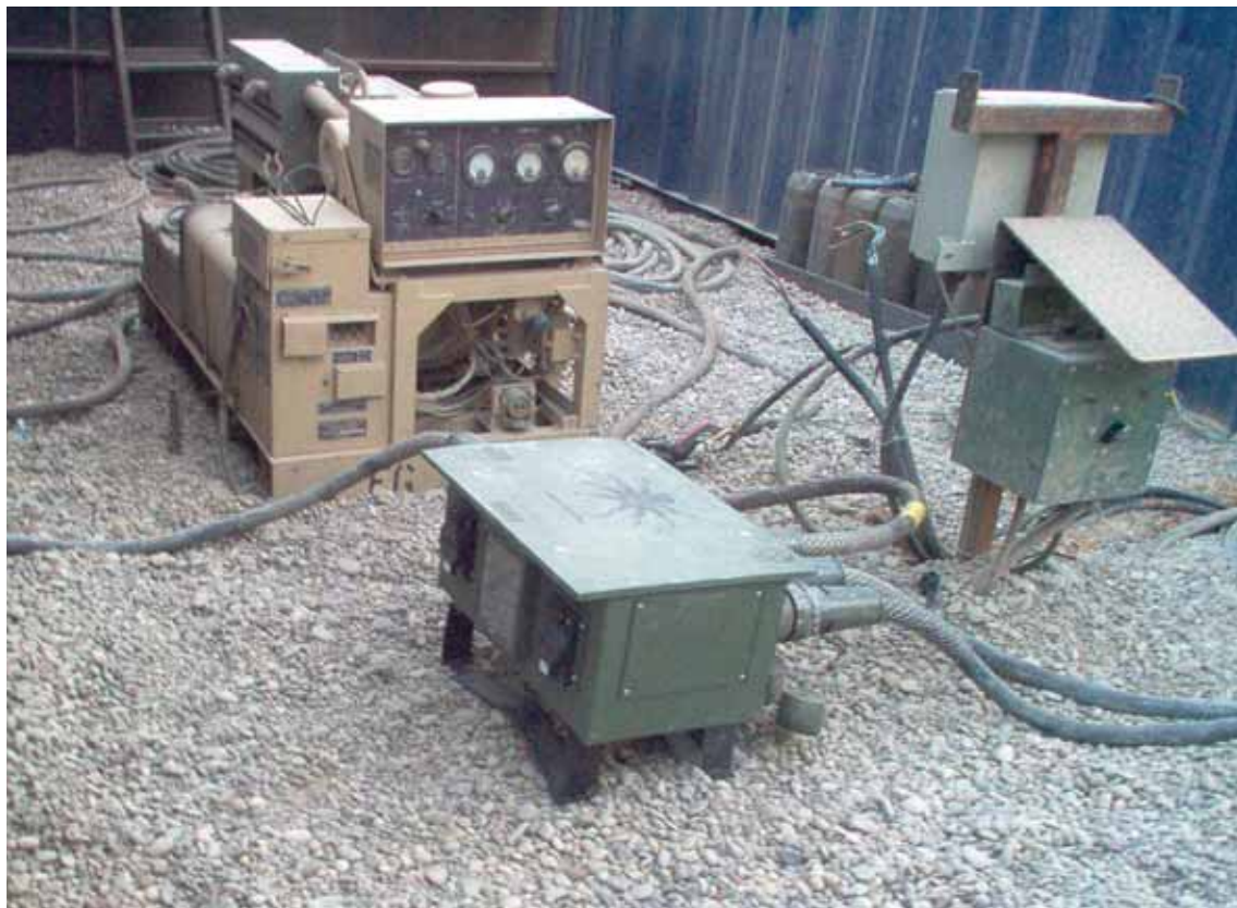
FOB/TOC Power Distribution (100 AMP) Using Mil Type 1068 Oscar™ Box
